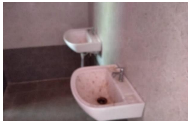
Conditions of one of the SS Restroom
